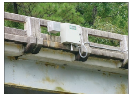
Figure 3. Stage can be measured using a non-contact radar stage sensor mounted on a bridge.
